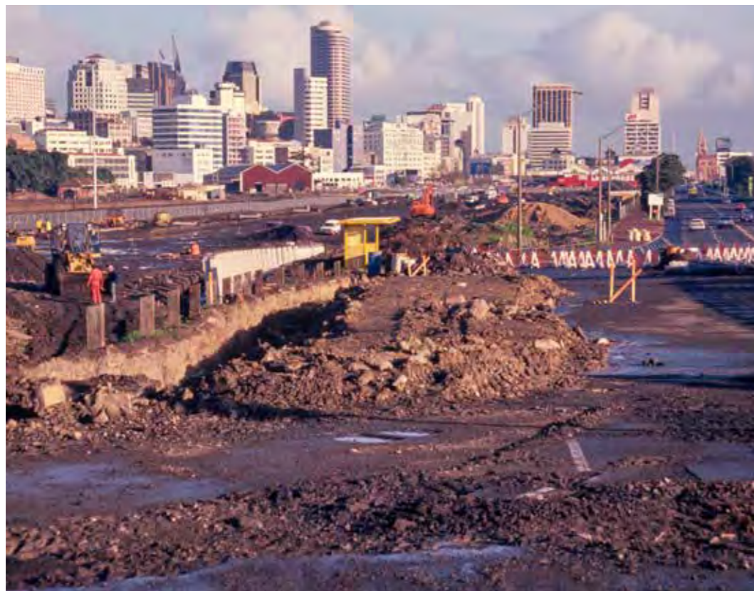
Britomart rail extension (1994), Auckland City Council – Sir George Grey Special Collections, Auckland Libraries 1108-26.
