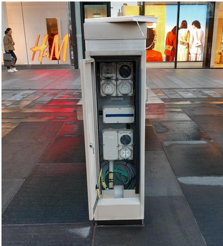
Figure 4: Photo of power box
